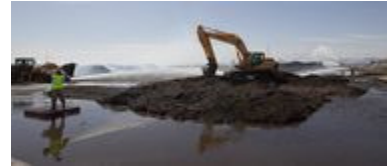
Workers spray water on smoldering compost piles on March 5 as tractors break the piles apart to allow the water to soak farther in.
